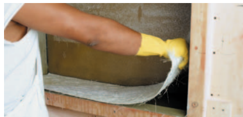
4. Individual layers of fiberglass are laid up and then wetted out with a fire retardant polyester resin.
