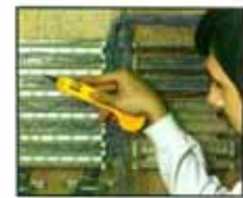
Trace phone/data wiring.
